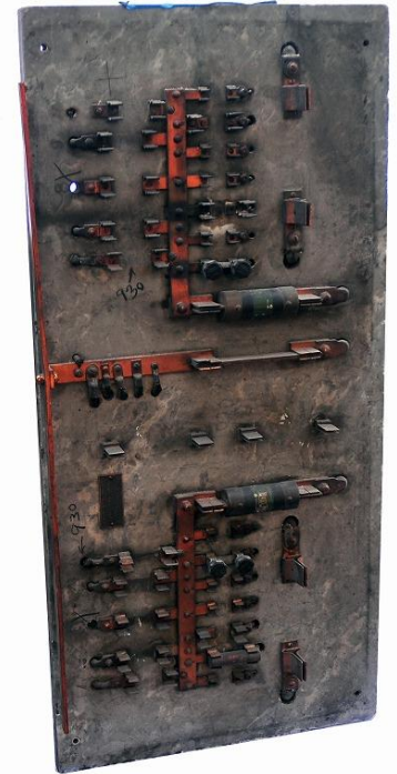
ELECTRIC FUSE SLATE H1070 W510 D90 3742-08-02 150,000
